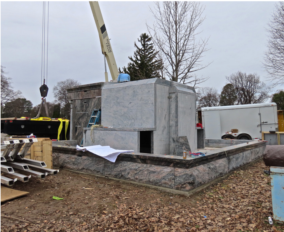
The interior walls were constructed first, and since these walls are vertical, the pyramid has a lot of unusable space. Photo by Richard Reisem.
