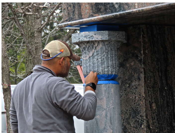
Egyptian Revival style capitals incorporate an acanthus-leaf motif. Notice that there is a space between the capital and the portico roof. To ancient Egyptians, this was intended to suggest that the column was not really holding up the roof. It was being held up by the divine power of the Egyptian sun god, Ra. Photo by Richard Reisem.
