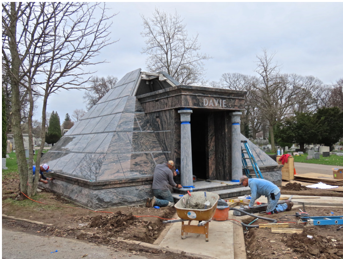
Three talented craftsmen constructed the mausoleum. From left: Randy Faulk, JP Saucedo, and Allen Kent, owner of A Kent Construction, Kempner, Texas. Photo by Richard Reisem.
