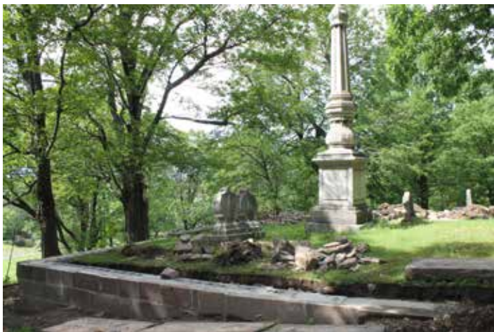
One of the summer construction projects includes the surrounding retaining wall of the Hunter/Carter Lot No. 57 in Section R just west of Nathaniel Rochester's gravesite.
